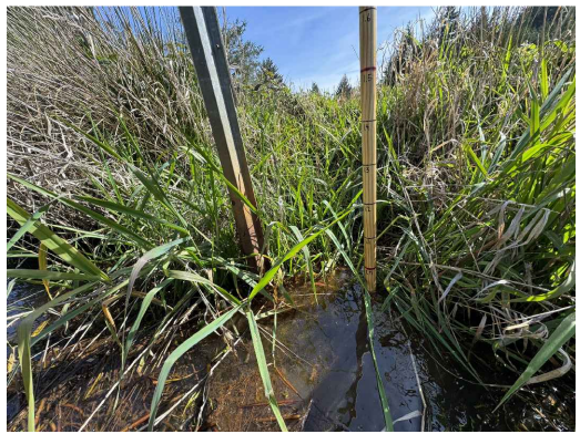
2 ALDERWOOD DRIVE CULVERT UPSTREAM INLET BURIED IN SEDIMENT Scale: NTS
