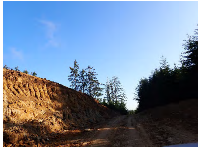
Cut slope along new road to be named in the southwest portion of property.
